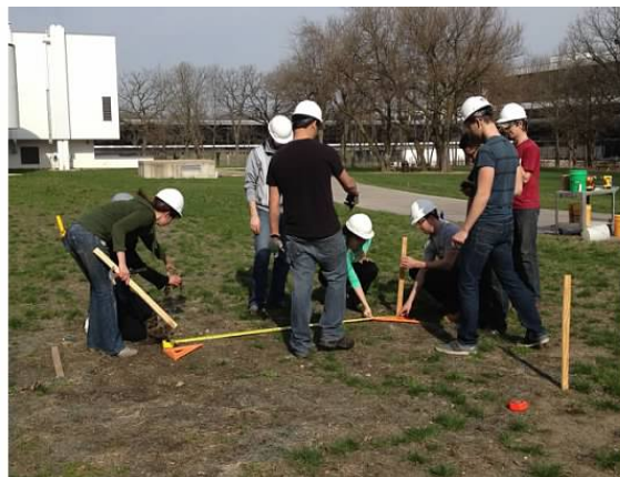
Figure 1.4: The photo below illustrates students staking out the site and measuring the outside perimeter of the pavilion, before the administration required the class to stop work.
