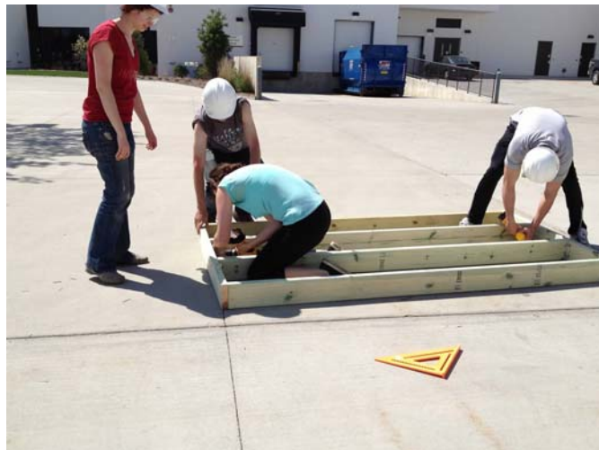
Figure 1.5: The photo below illustrates students building in the second approved location, and the construction of the wood framing floor system on grade.
