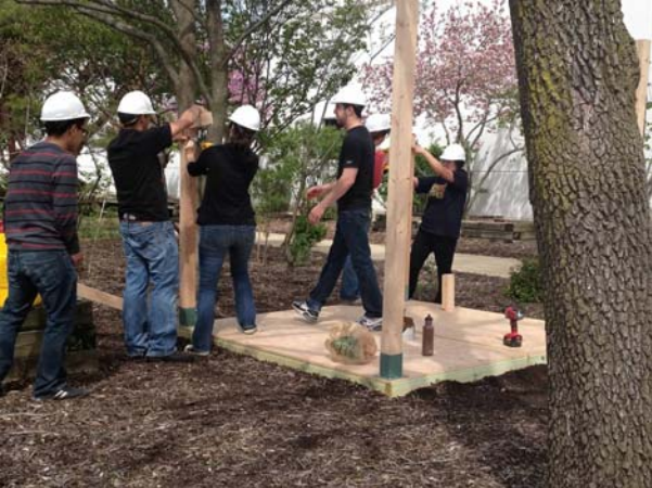
Figure 1.7: The photo below illustrates students working on the floor and wall framing to create the pavilion.
